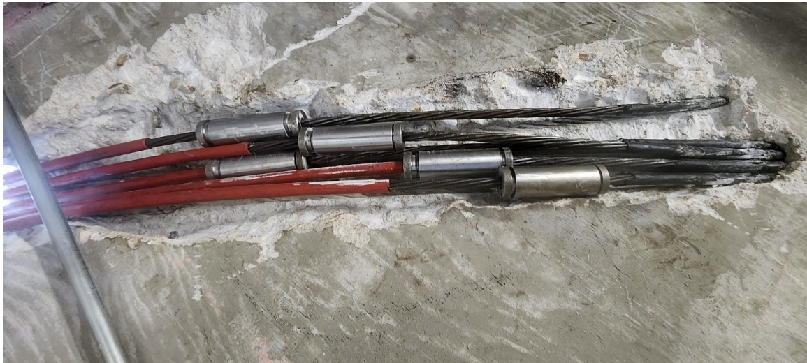
Photo: Installation of these splice couplers within the tendon sweep places an eccentric load on the hardware.
